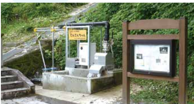
Small-scale hydroelectric generation facility using agricultural water (Yotsuya district, Shinshiro City)
