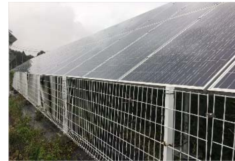
(不適切な柵塀設置の事例)
